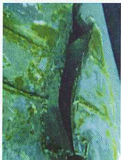
Hydrex recently sent a nine-man team to the United Arab Emirates to repair the shell plating of a bulk carrier that indented after a grounding and subsequently cracked.
